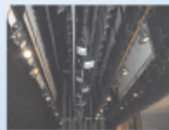
Theatrical Dimming & Lighting Fixtures
